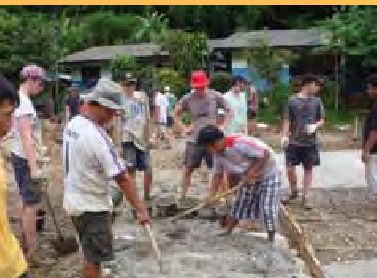
Giving globally: Power of 9 students assist with building a concrete assembly area in a hill-tribe school in north west Thailand.
